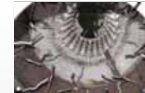
Refractory Lined Expansion Joint
